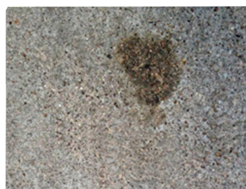
Oil on concrete before treatment
